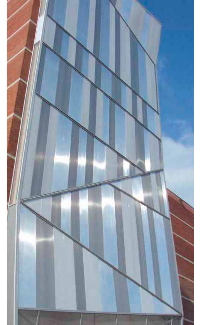
■ Fitting contractor: ATV Design, Houilles (78) - Tel: 06 26 04 44 78. Cladding Danpalon 16 MC 600 and 1040 Crystal, Opal and Aluminium.
